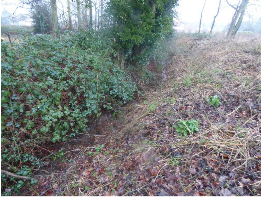
Photograph 7 – Wet ditch along the southern boundary of the site.
