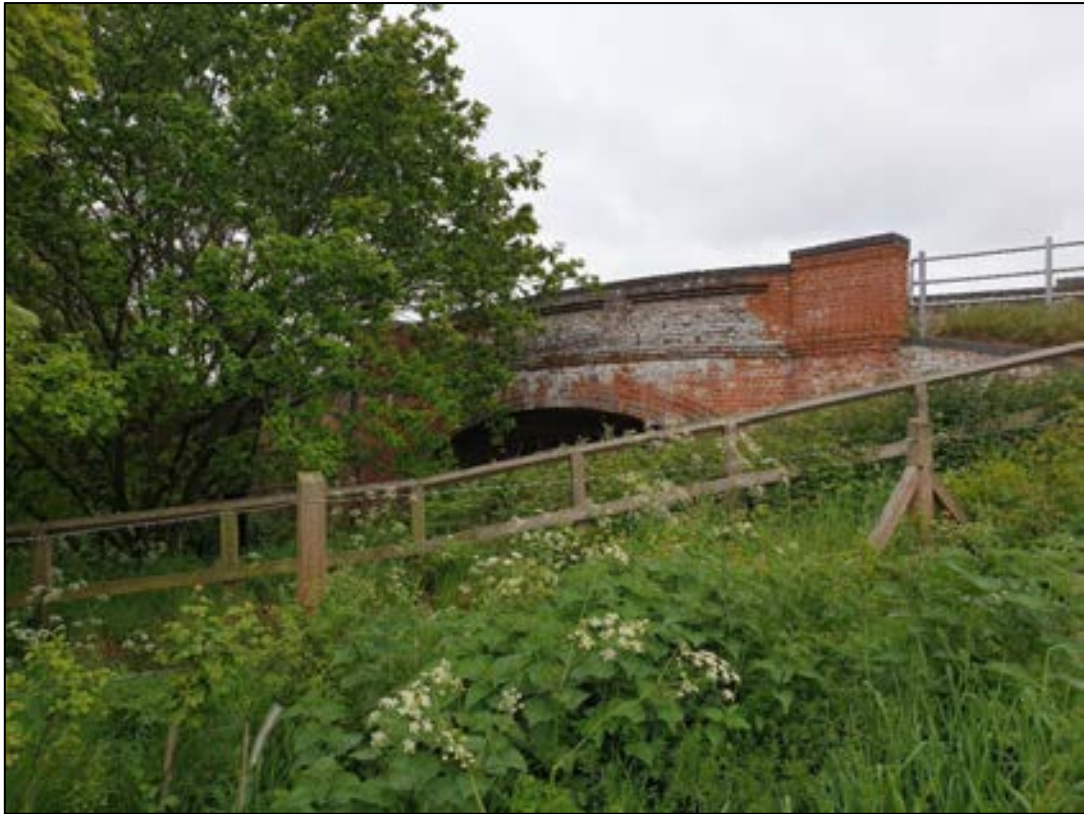
DP 25. View west of former railway bridge within the proposed development site.
