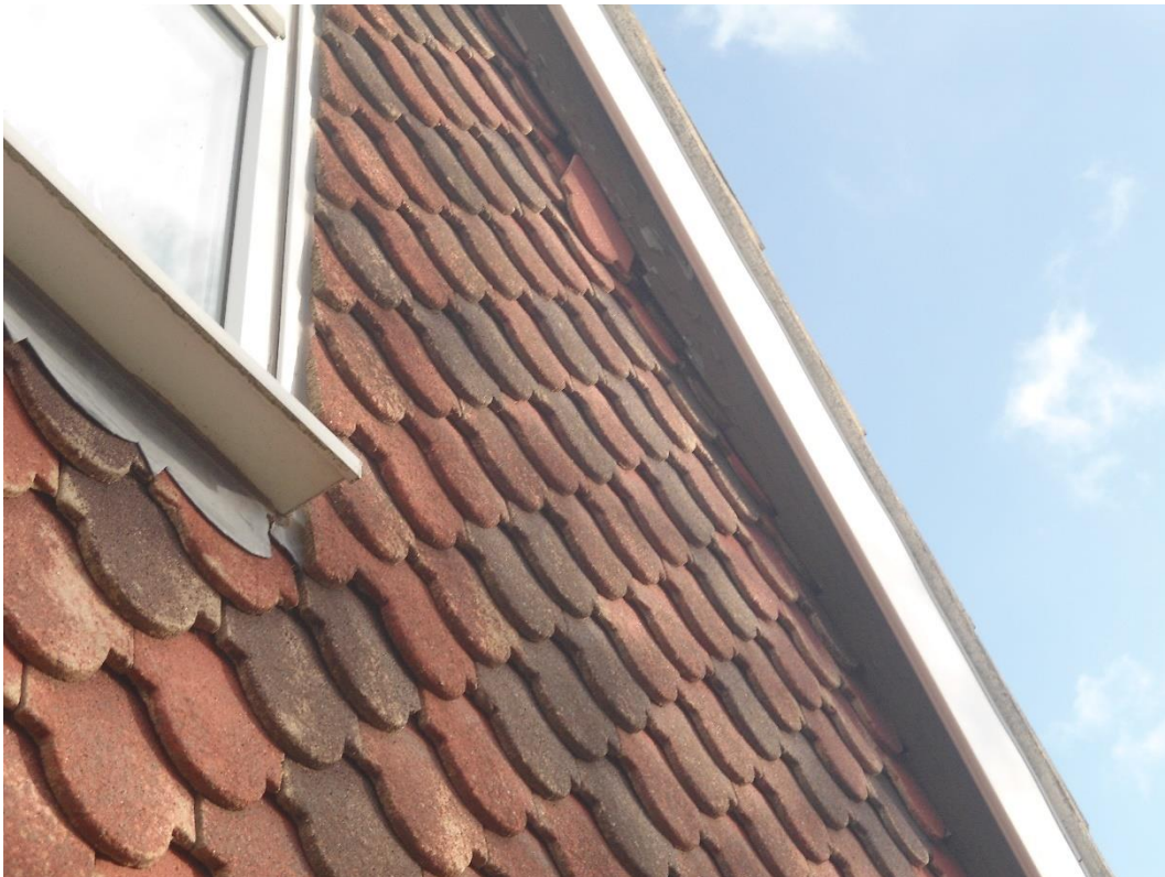
Photo 34: Western elevation showing cavities in the soffits which could potentially be used by roosting bats
