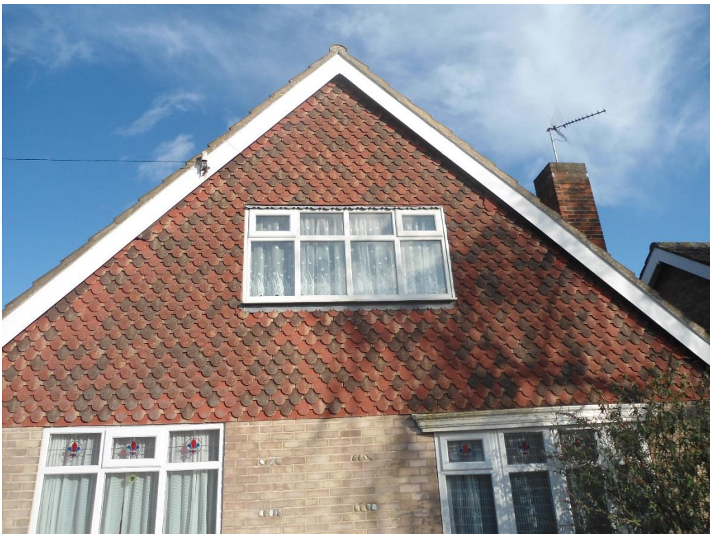
Photo 32: View of the western elevation of 3 Prince Andrews Road showing tight fitting tile cladding
