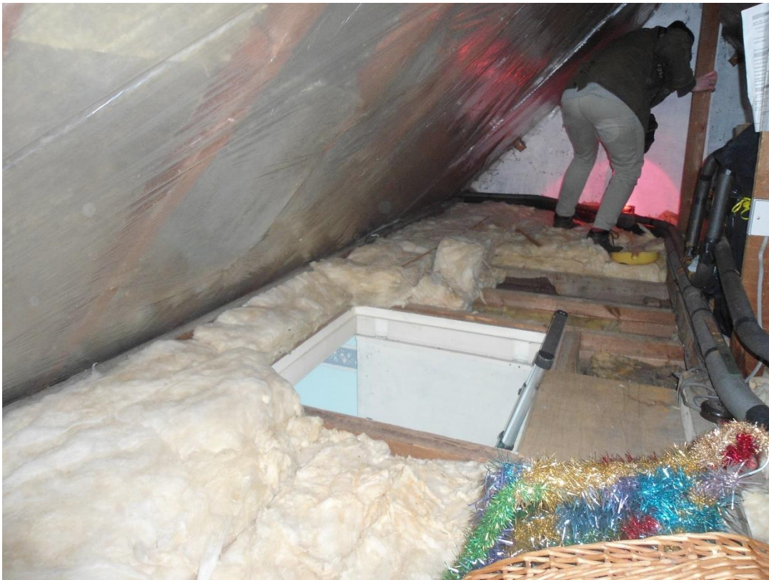
Photo 37: View of the roofspace, heavily insulated with plastic film covering bitumen lining and modern machine timbers
