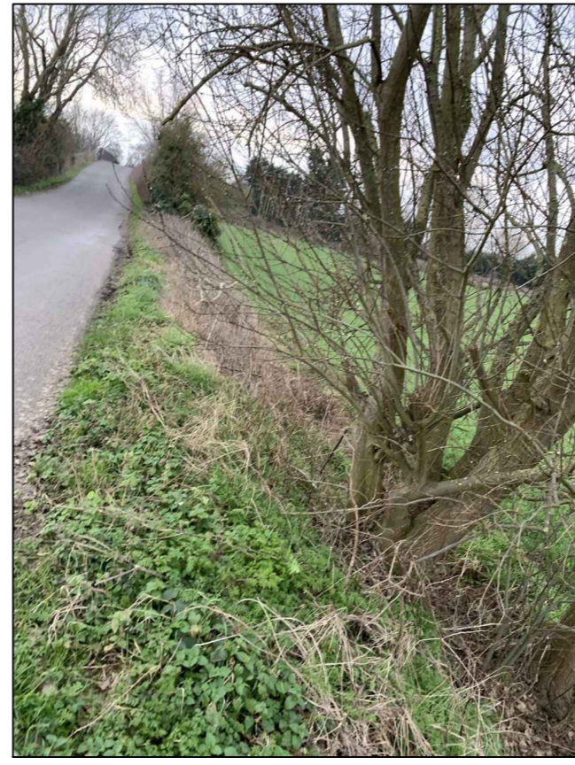
Approximate start of transition to bridge slope. Steep embankment down to adjacent field from this point.
