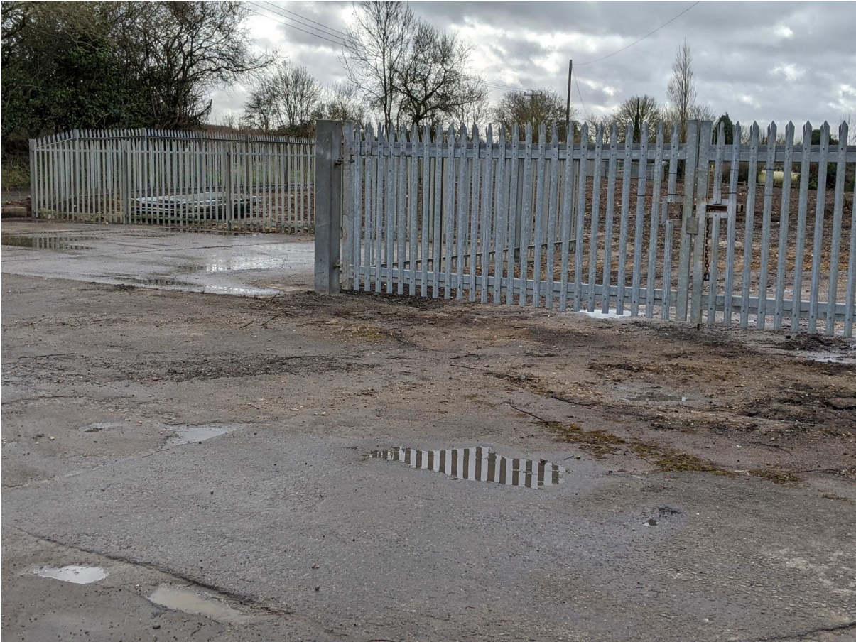
f) Entrance gates to cleared site. It appears that the concrete base here could be shared with GCP.
