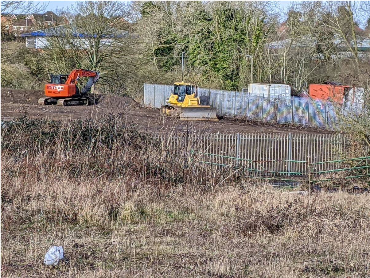
e) Clearer view of perimeter fencing to the right of site, to Gary Cooper Paving.
